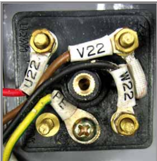
Figure 79. Pump motor (M2) wiring.
