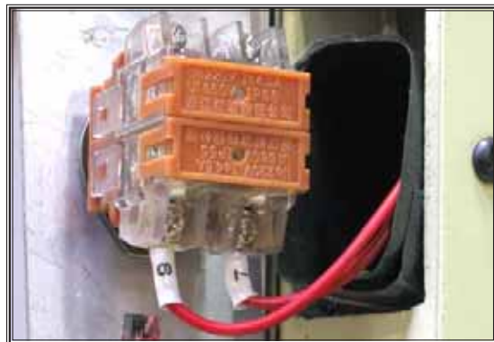
Figure 85. Pump switch (SA2).
