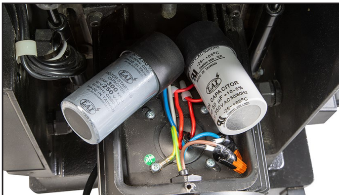
Figure 76. Main motor capacitor wiring.
