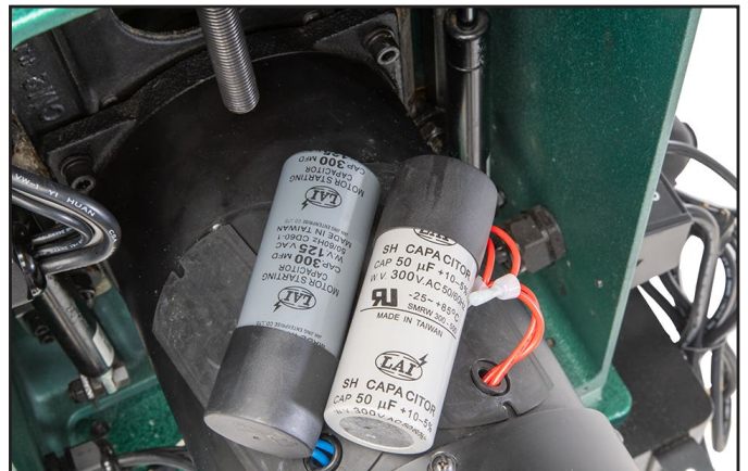
Figure 68. Main motor capacitor wiring.
