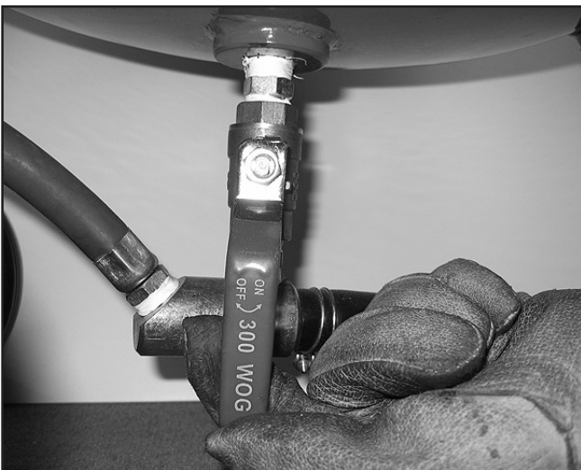
Figure 14. Sand metering valve in the full-open position.
