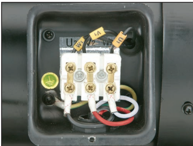
Figure 5. Motor junction box wiring.
