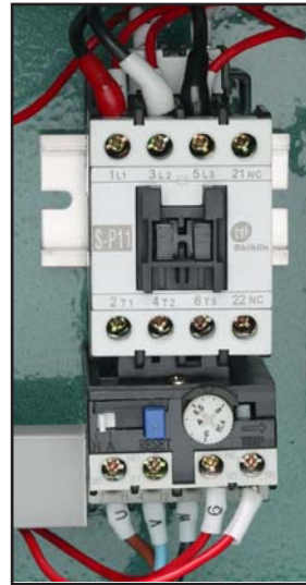
Figure 49. Contactor and thermal relay.
