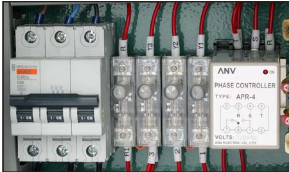
Figure 44. Input relay, fuse bus, phase controller.
