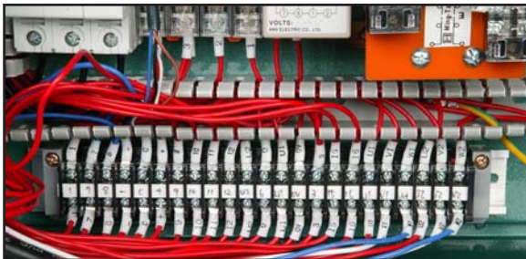
Figure 46. Main terminal block.
