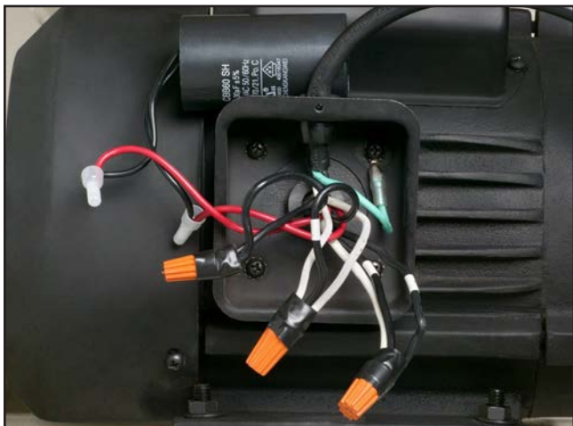
Figure 66. Motor junction box and capacitor wiring.
