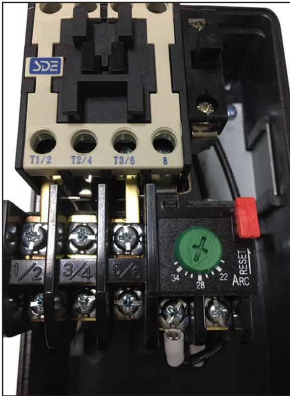
Figure 46. G0671 MA-15 contactor.
