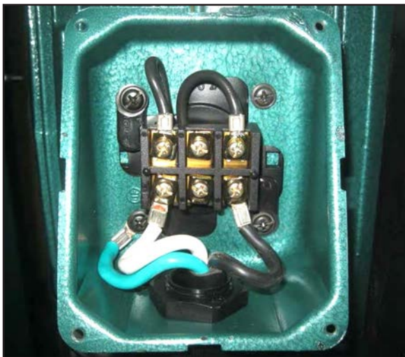
Figure 47. G0671 motor junction box.
