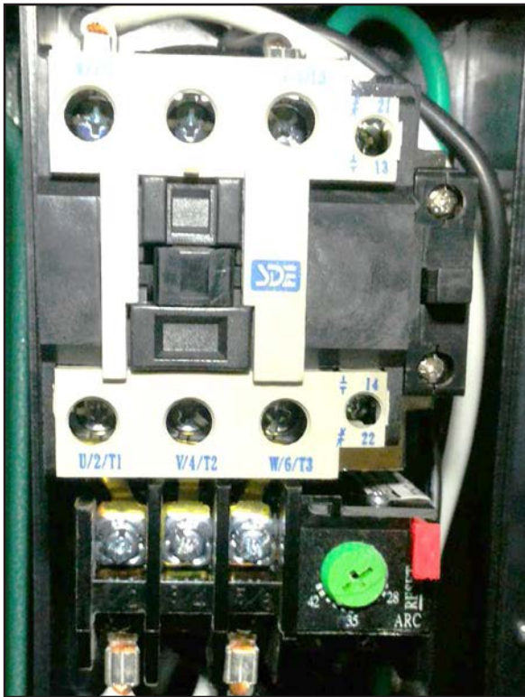
Figure 48. G0672 MA-30 contactor.
