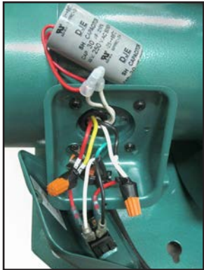
Figure 31. 120V junction box.
