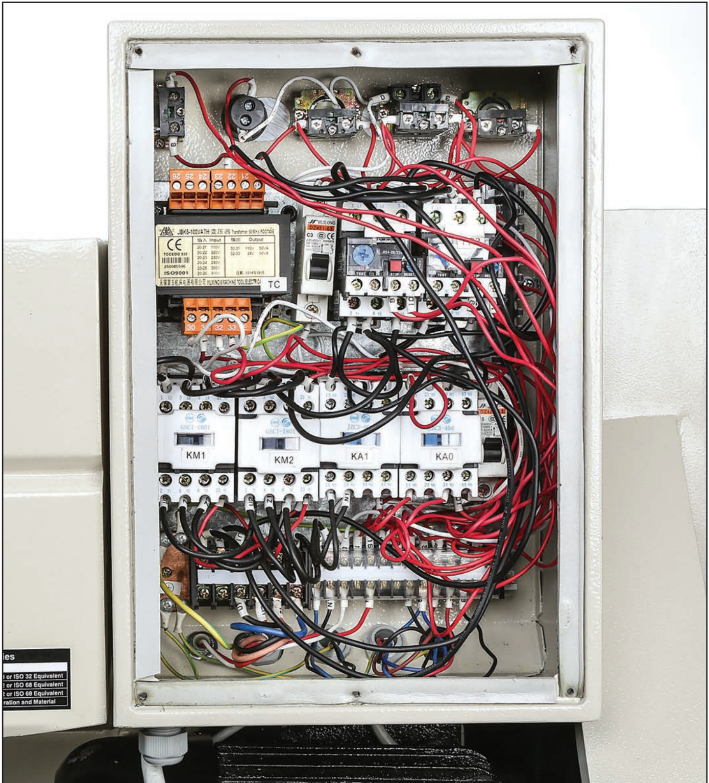
Figure 142. Control panel wiring.
