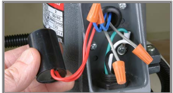
Figure 46. Pump motor/capacitor (M2).
