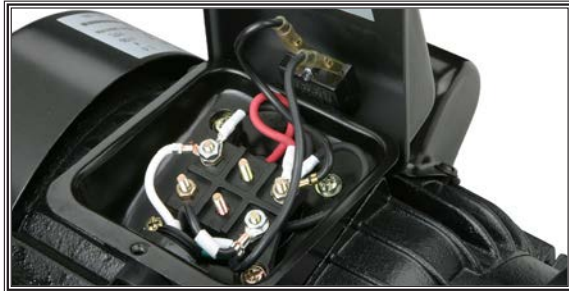
Figure 42. Junction box (M1).
