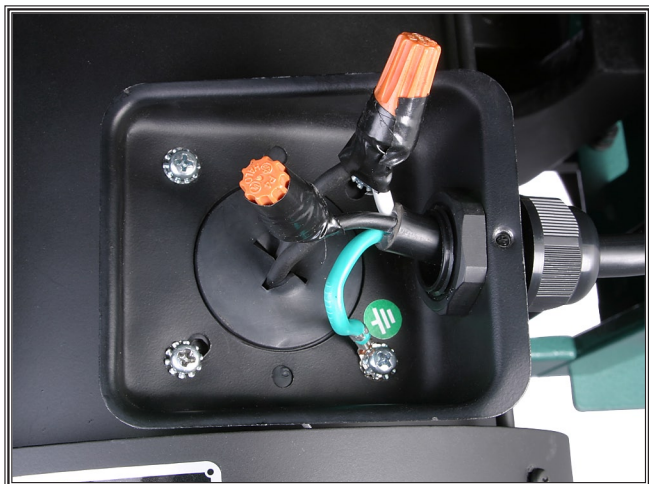
Figure 78. W1761 motor junction box, 220V single-phase.
