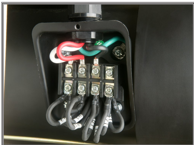
Figure 79. W1762 motor junction box, 220V 3-phase.
