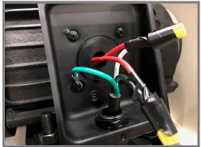
Figure 65. W1864 motor junction box.
