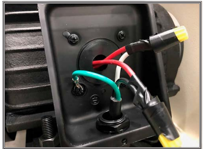
Figure 69. W1865 motor junction box.
